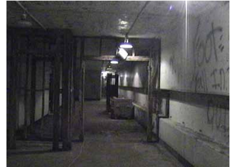
Standing around the center of the battery looking towards Gun Block 2. These are the remnants of one of the rooms that the Navy added after the war.
