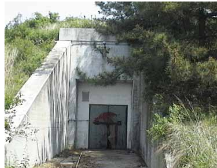
The center rear entrance of Battery 519 before the trees were cut down and the doors were replaced.
