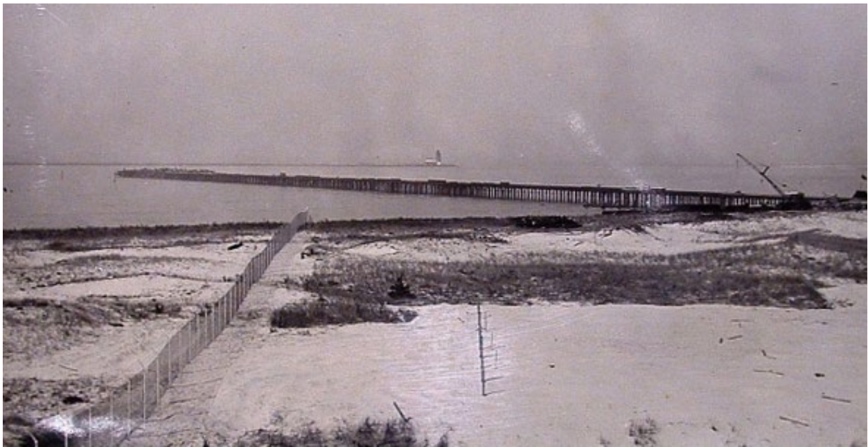
Construction is nearly complete on the Fort Miles pier built as part of the Mine Command operation. U.S. Army ships docked at the pier and mines were loaded by fort personnel. It's now the Cape Henlopen State Park fishing pier. STATE PARK PHOTO
