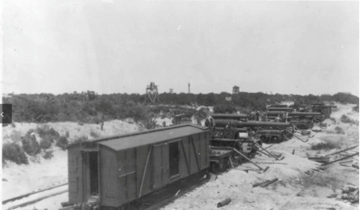
Trains supplied most of the materials needed to construct Fort Miles, starting in 1941. STATE PARK PHOTO
